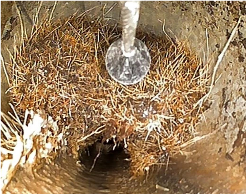
Roots Ball Barrell from 7 o'clock to 5 o'clock, 80% lost.
