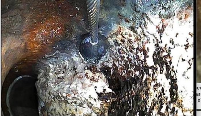
Deposits Attached Encrustation, 25% of cross-sectional area from 4 o'clock to 10 o'clock.
