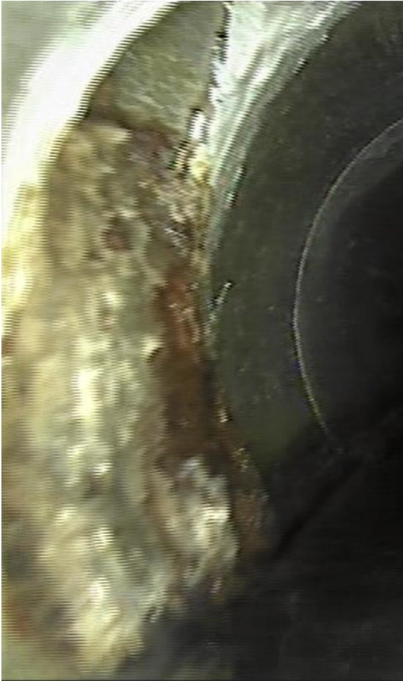
Deposits Attached Encrustation, 75% of cross-sectional area from 9 o'clock to 11 o'clock.
