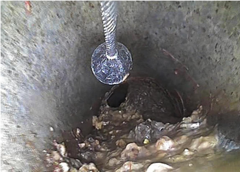
Roots Ball Joint from 1 o'clock to 8 o'clock, 65% lost.
